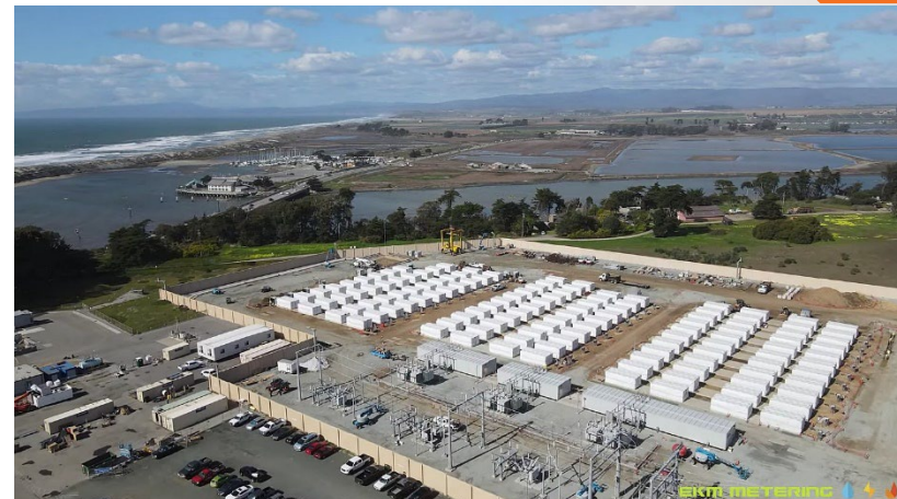
Moss Landing, California Tesla Megapack Battery Farm
